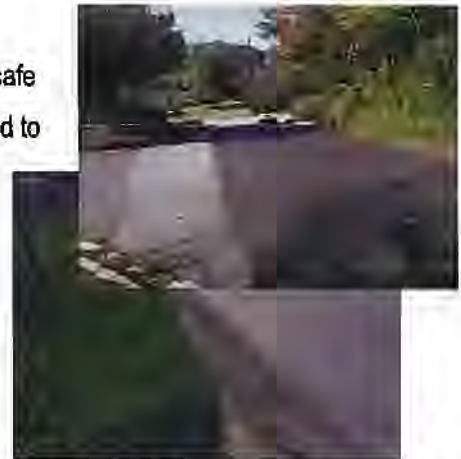
Photos 2 and 3: Existing conditions include a lack of sidewalks and limited shoulder widths with uneven pavement and drainage issues.
